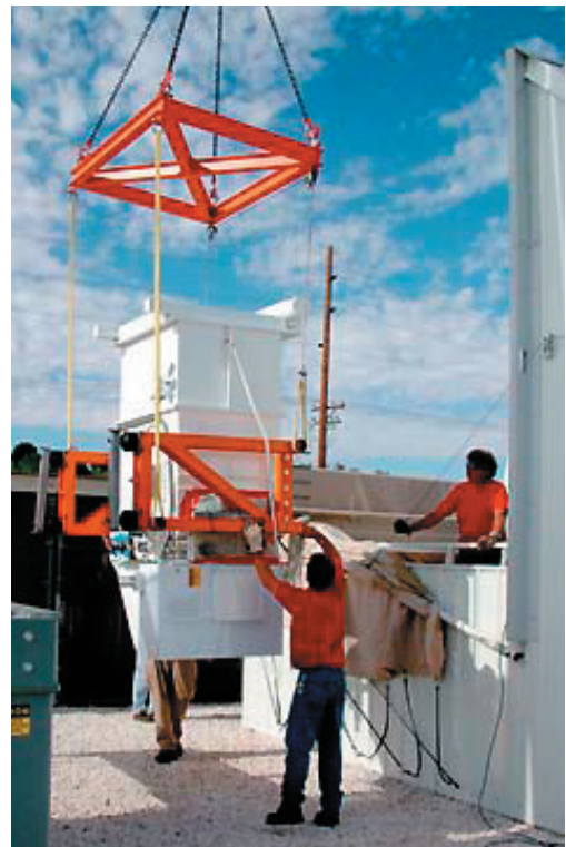
The SOLIS VSM instrument being repositioned for installation on the mount.
