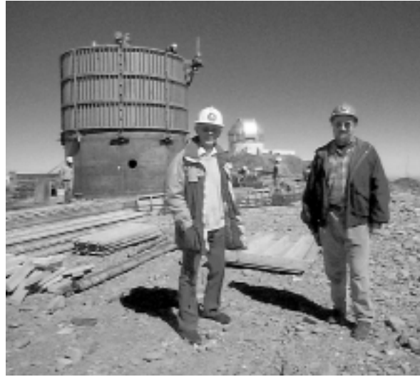
Malcolm Smith and Steve Heathcote stand in front of the pier that will support the SOAR telescope. In mid-April 2000 the concrete work for the lower half is complete, with the forms in place to the full height of the pier. The Gemini South dome is seen in the background.
